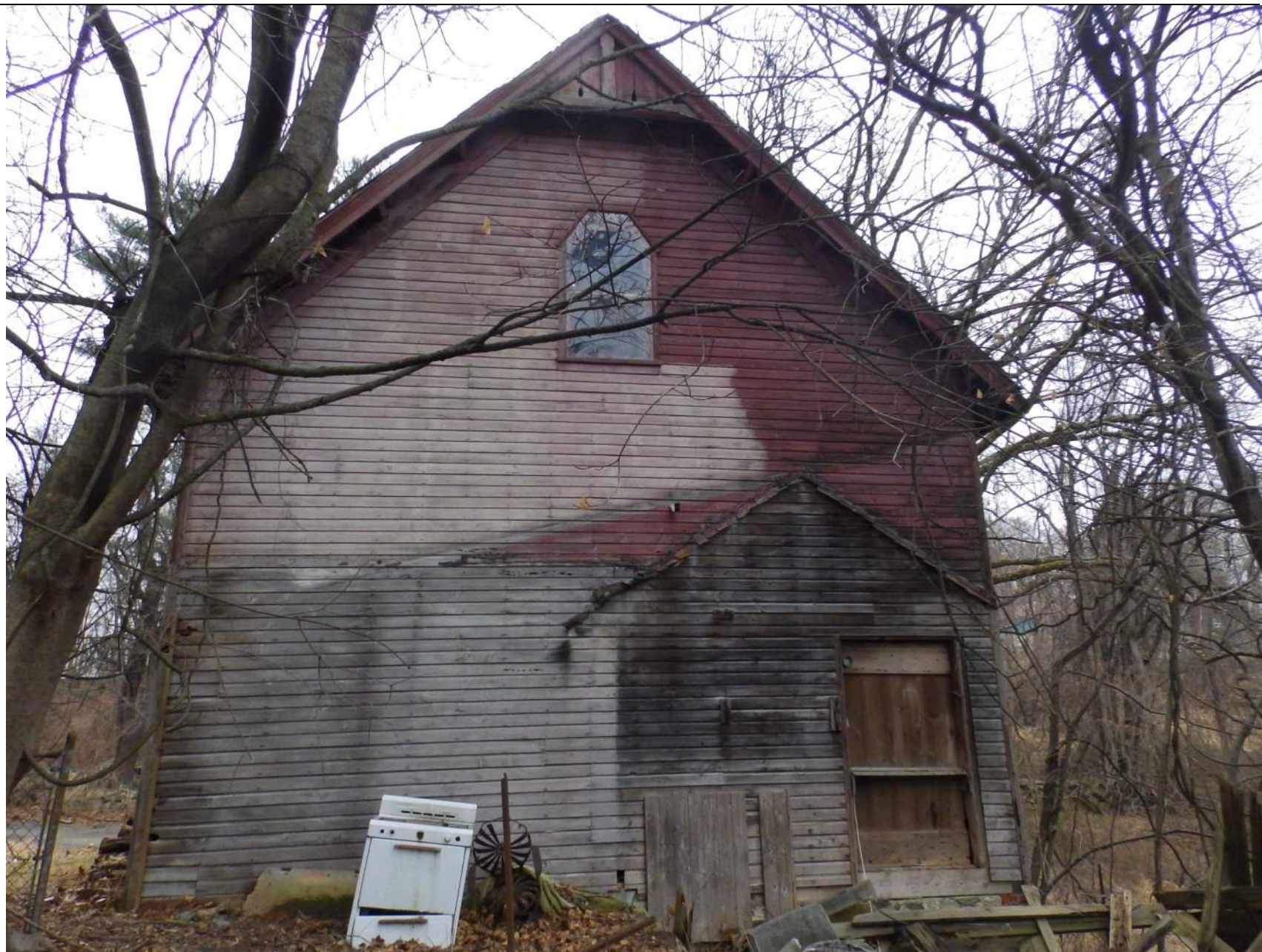
17. Western elevation of the Barn. Pool house addition has detached and collapsed.
