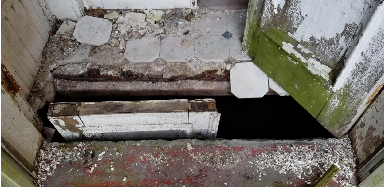
9. Portion of missing floor at main entry vestibule
