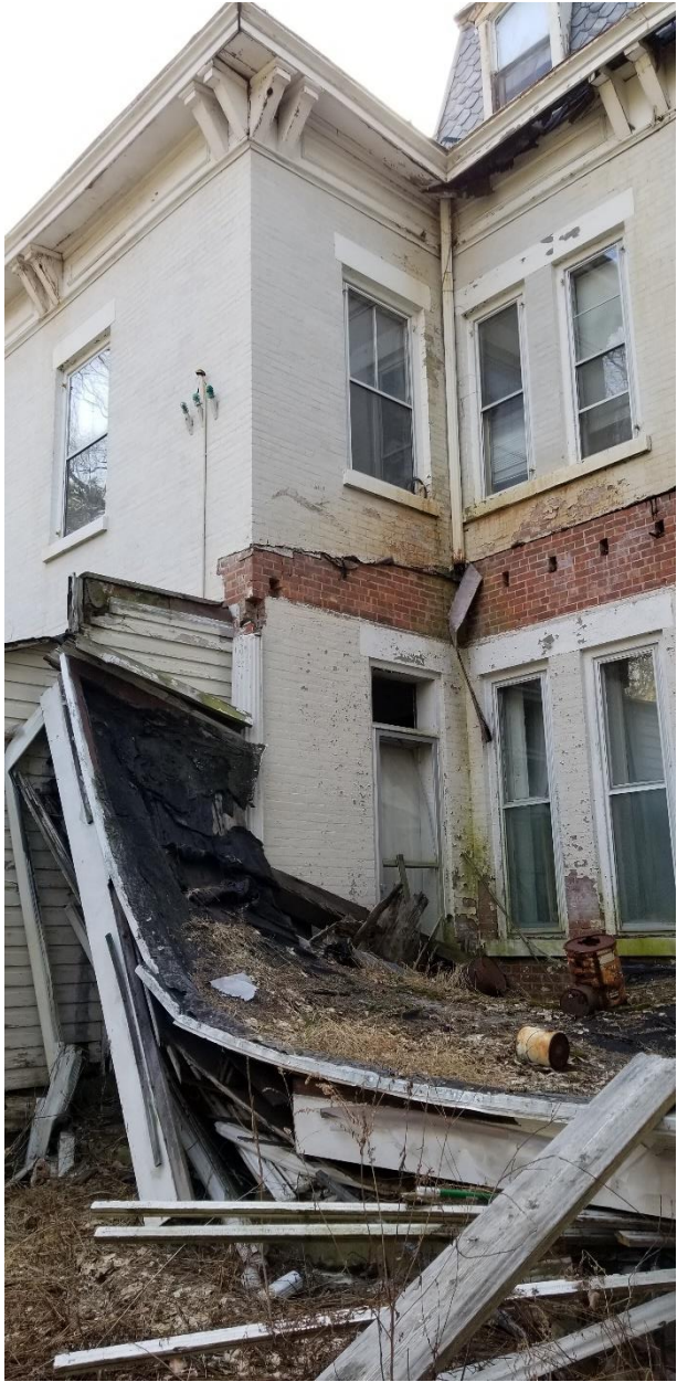
17. Collapsed porch roof on east elevation with debris
