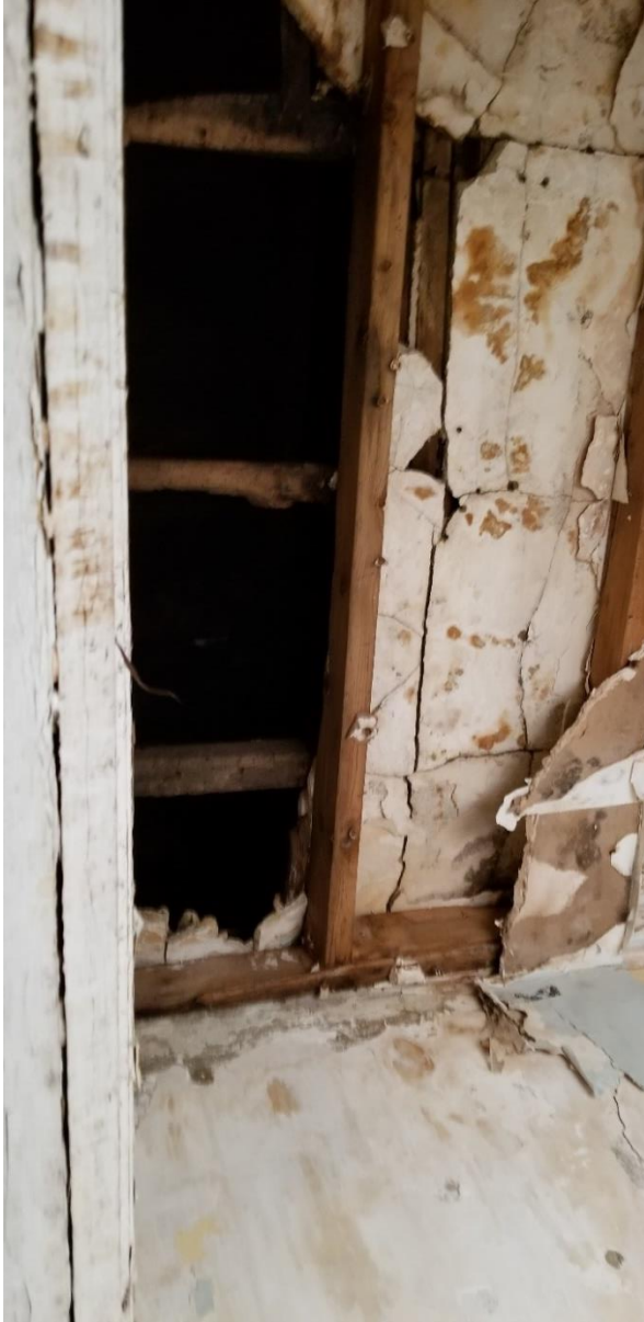
29. Ceiling damage due to leaking roof
