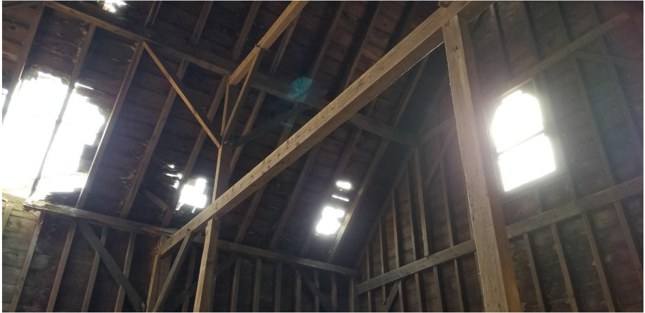
36. Damage and missing portions of existing roof
