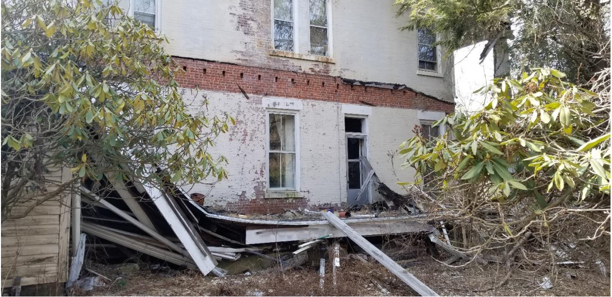
19. Collapsed porch roof on south elevation with debris
