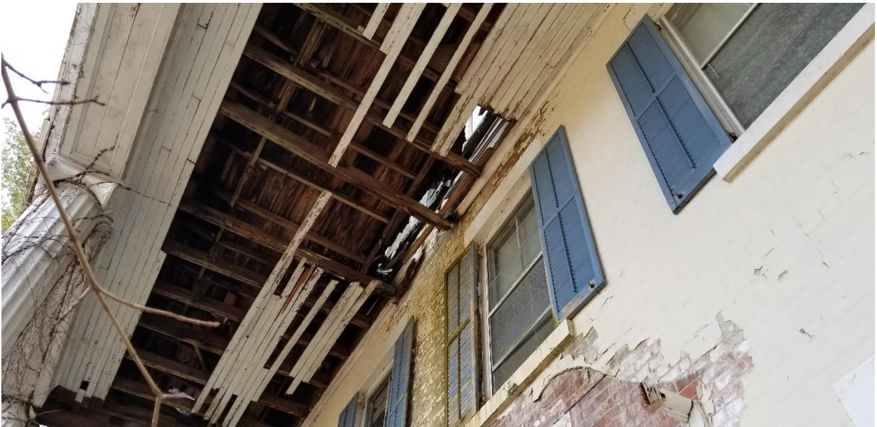
4. Deterioration of portico roof at front (north) elevation
