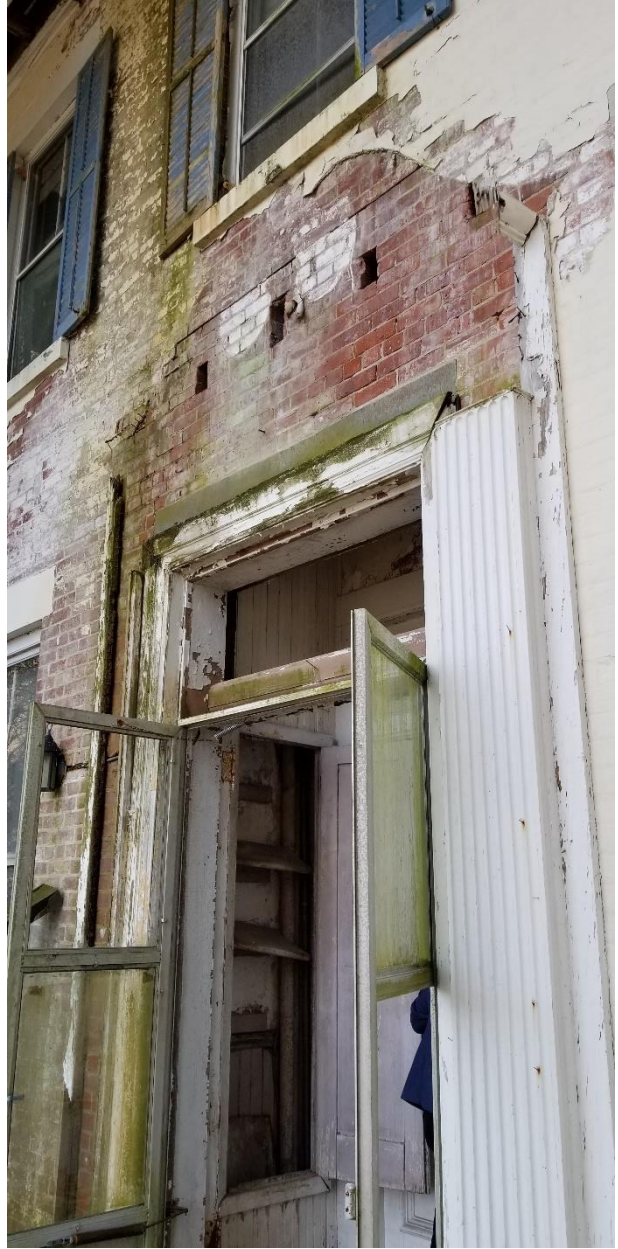
6. Missing decorative elements at front door
