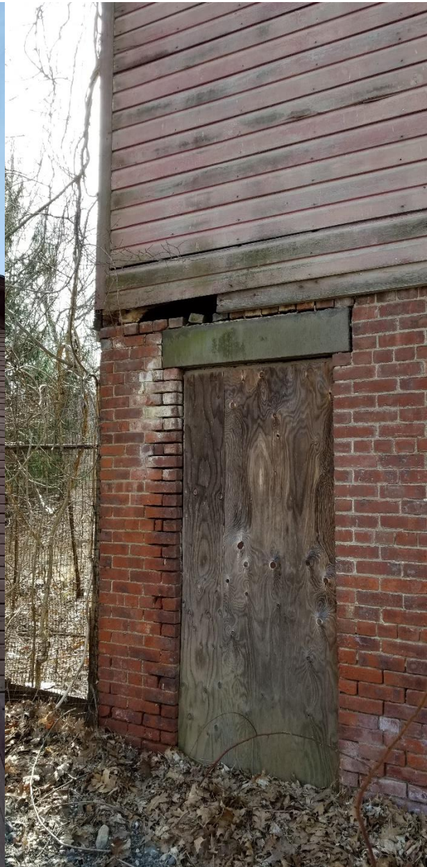
35. Deterioration to existing brick foundation
