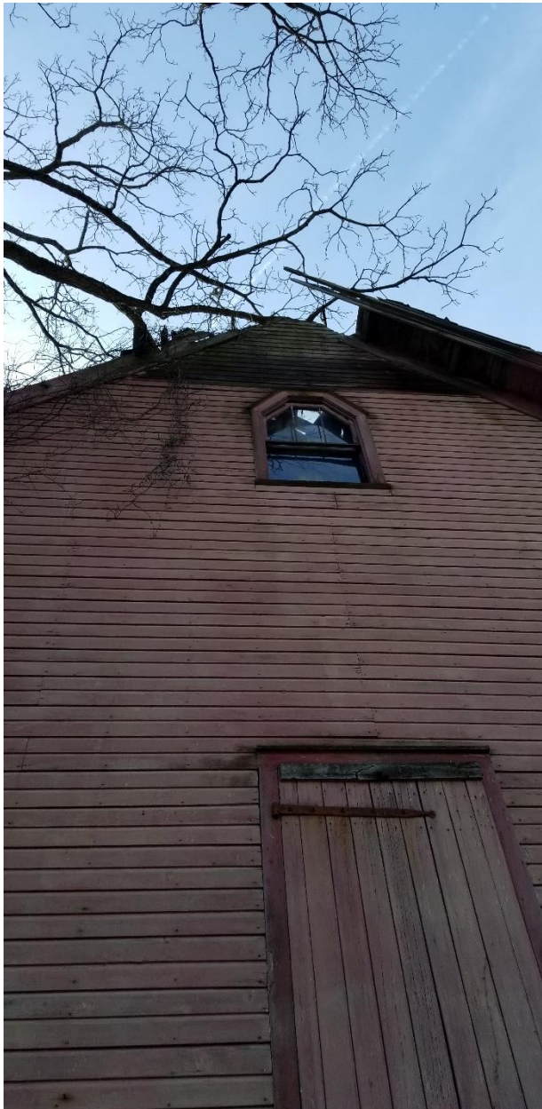
34. Deterioration and damage to eastern end of roof
