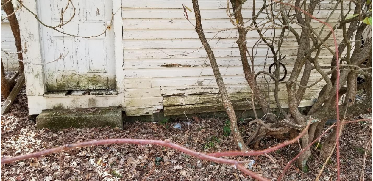
20. Deterioration of building addition area on southeast portion of structure
