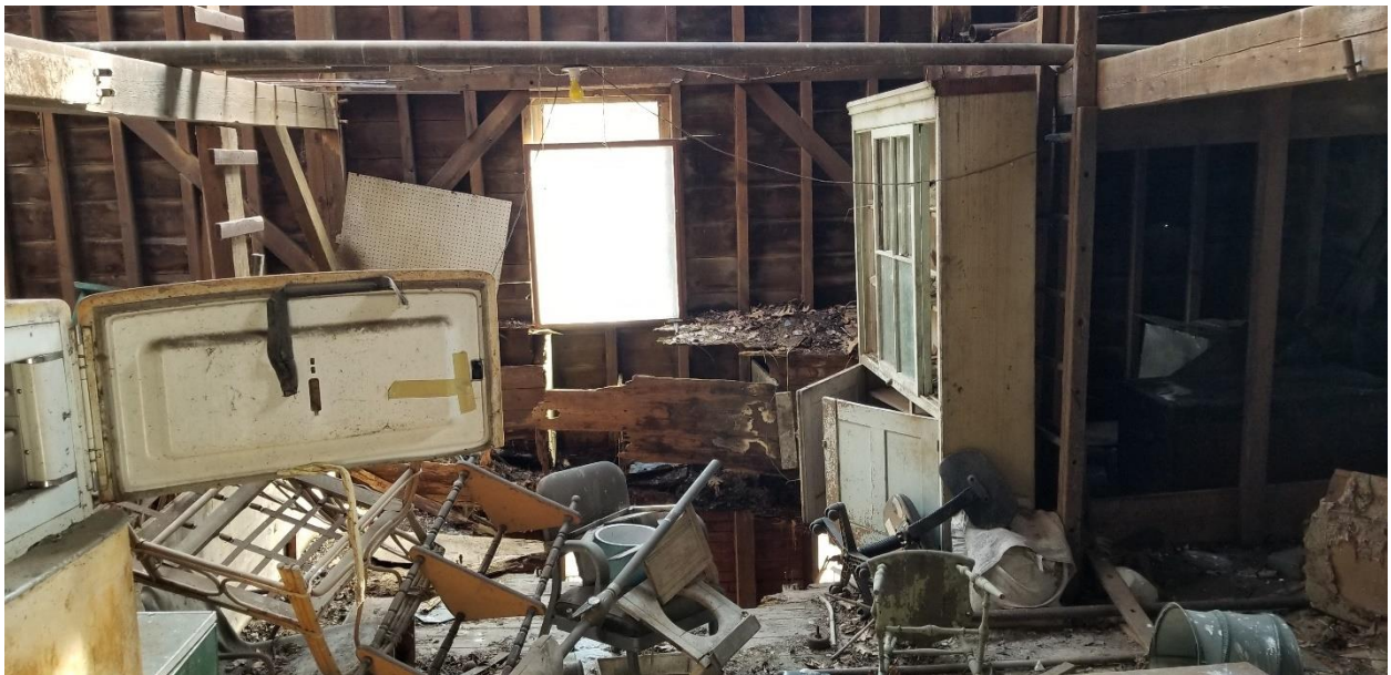
41. Collapsed floor on southern portion of barn
