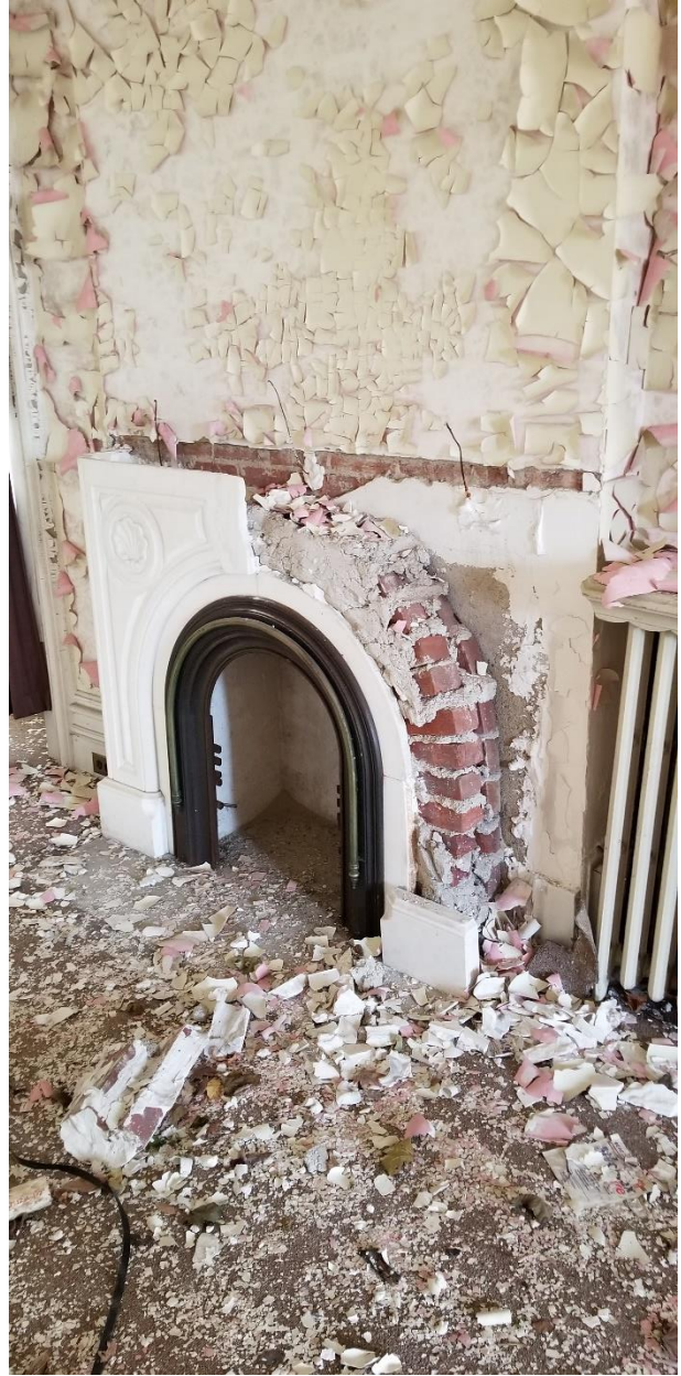
24. Existing damaged fireplace mantle
