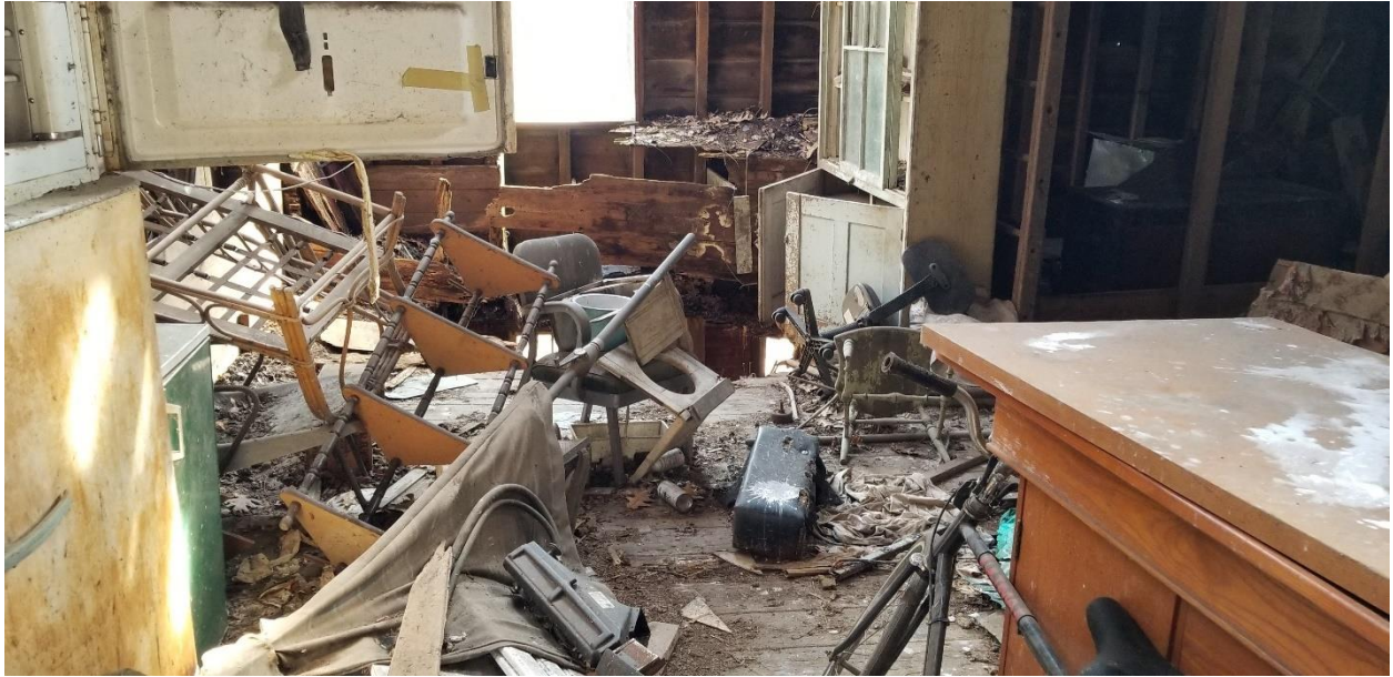
40. Collapsed floor on southern portion of barn
