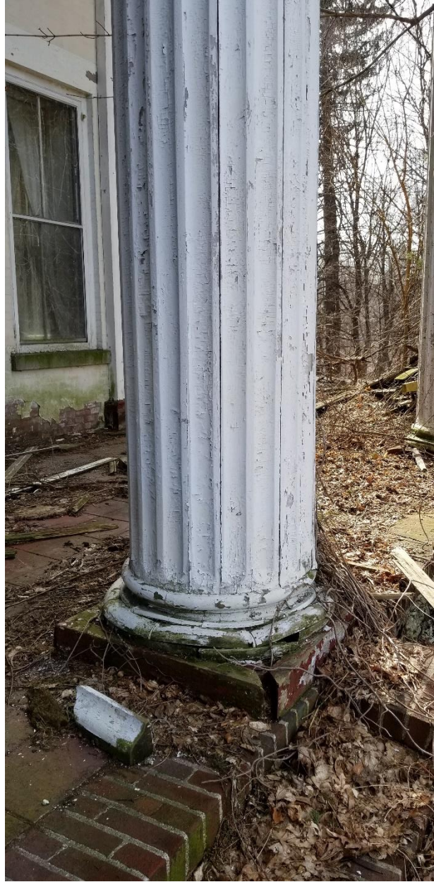
8. Deterioration of column base at front (north) elevation
