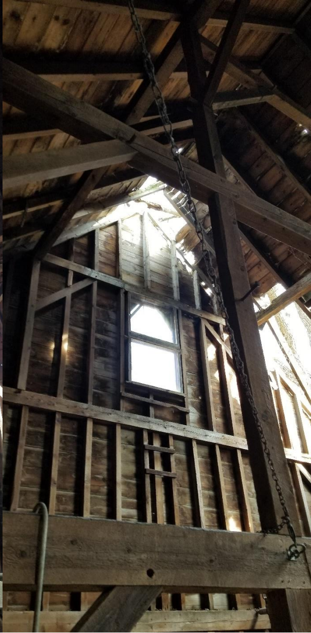
39. Missing sections of roof
