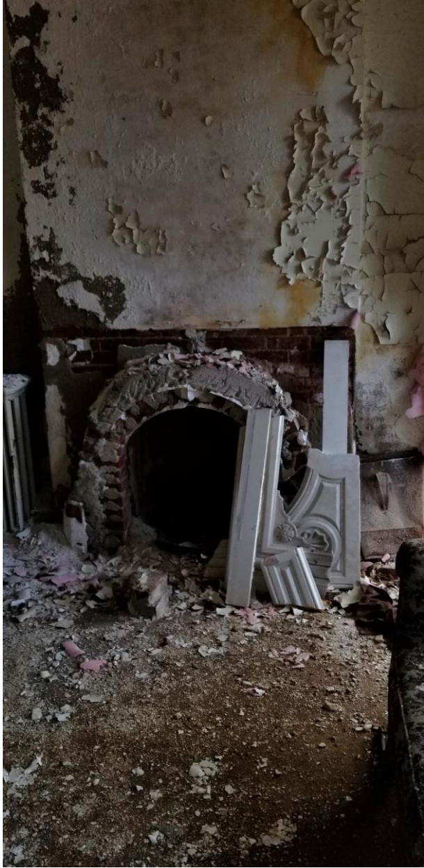
23. Existing damaged fireplace mantle
