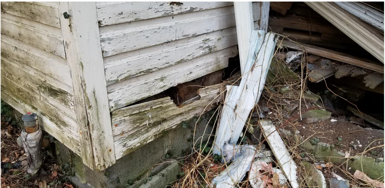
22. Deterioration of building addition area on southeast portion of structure
