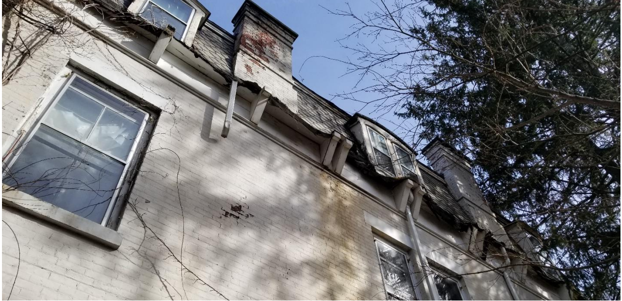
12. Deterioration of cornice
