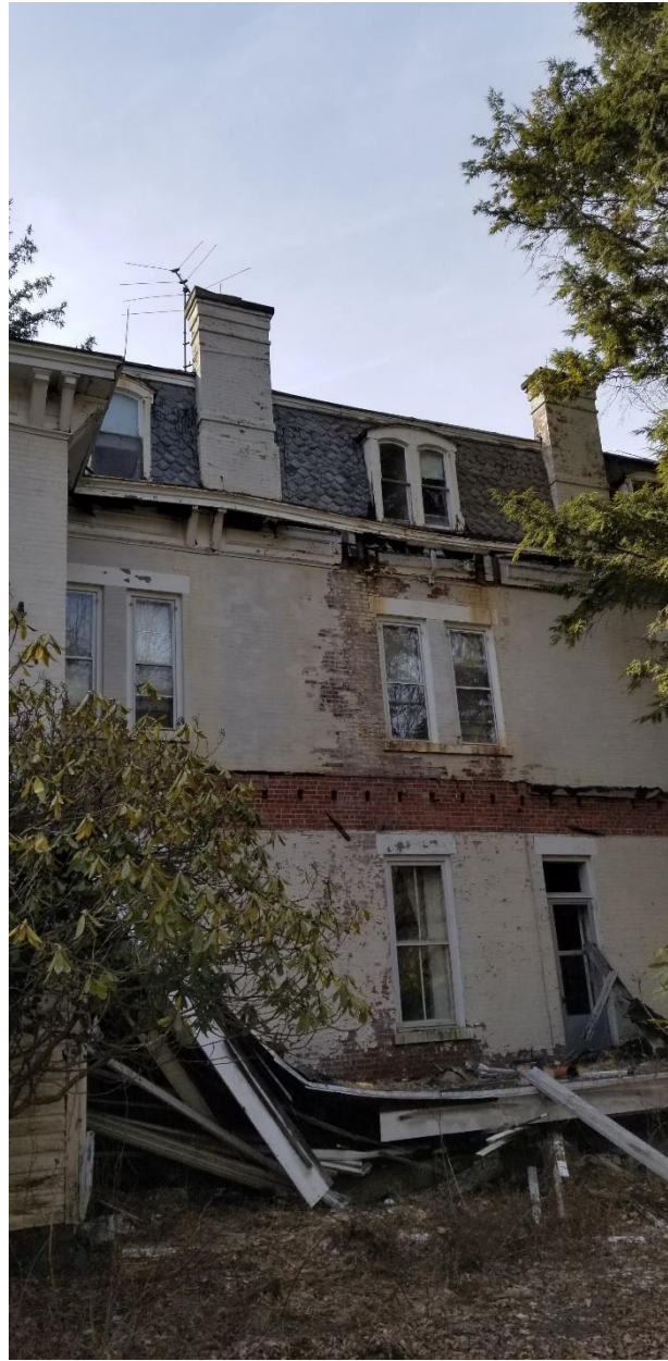
18. Collapsed porch roof on south elevation; debris
