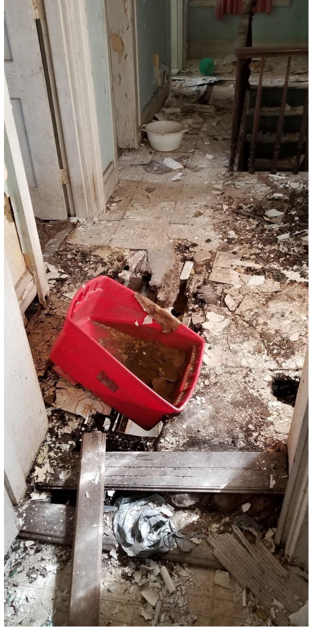
28. Missing floor over kitchen area, water collection from leaking roof, damage to structural components
