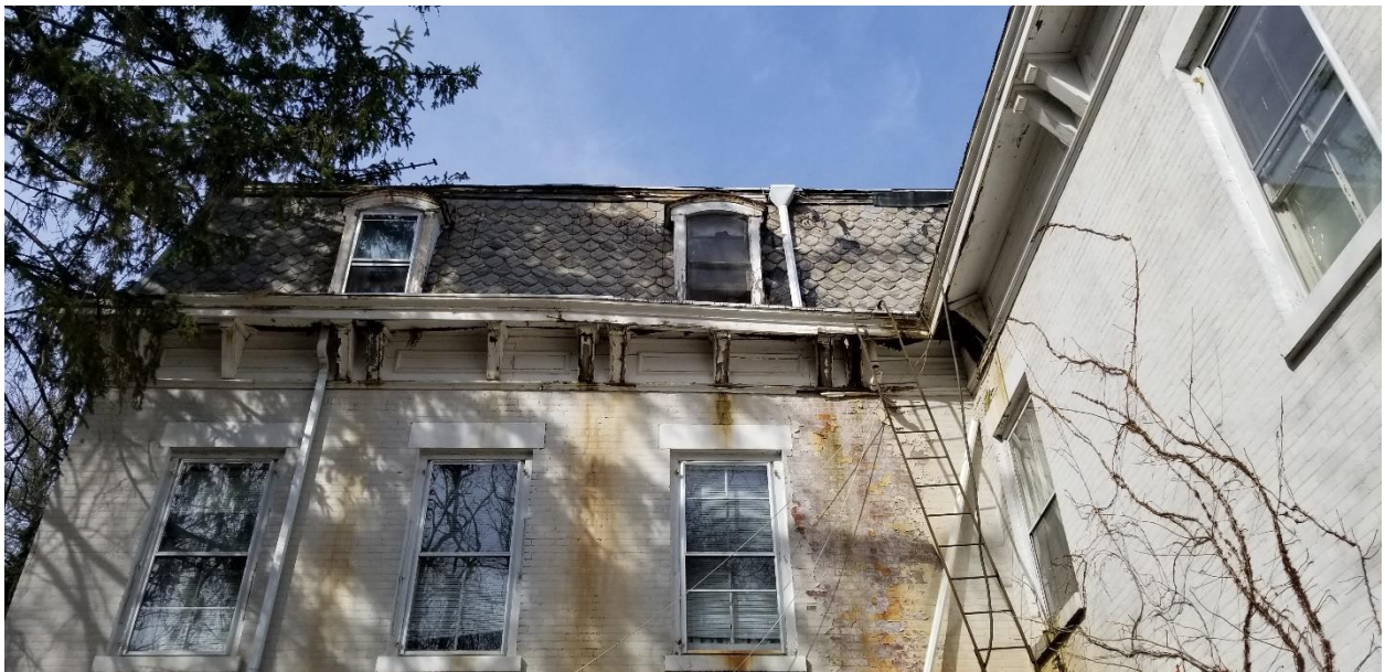
13. Deterioration of cornice and roof shingles; failure of gutter system
