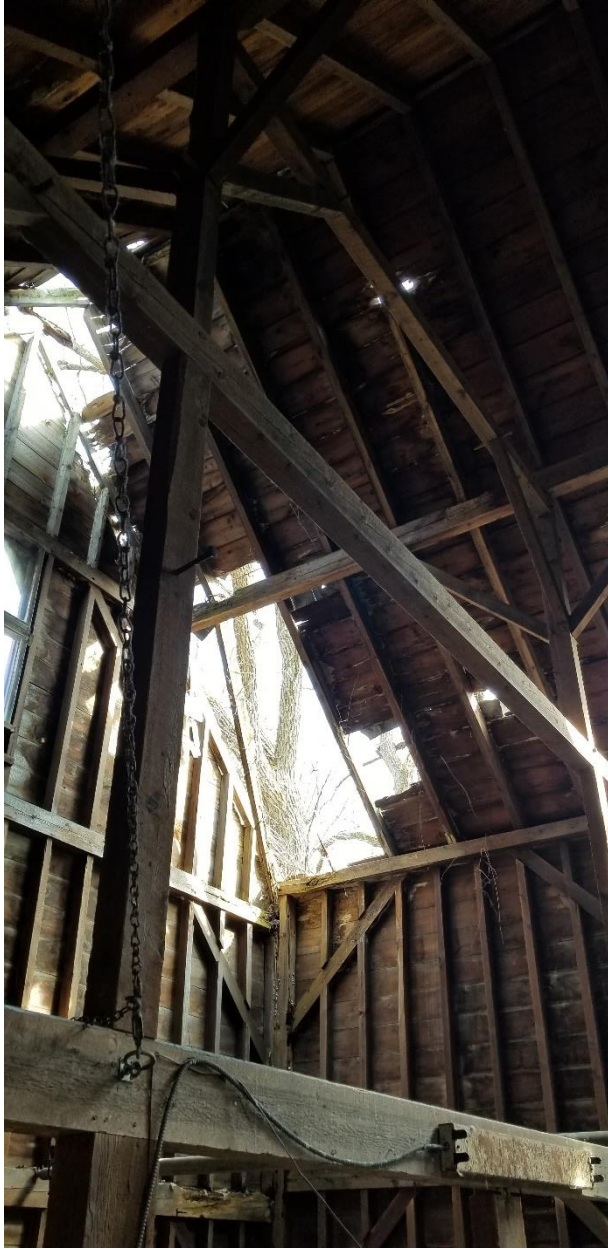
38. Deterioration and damage to roof and structural components
