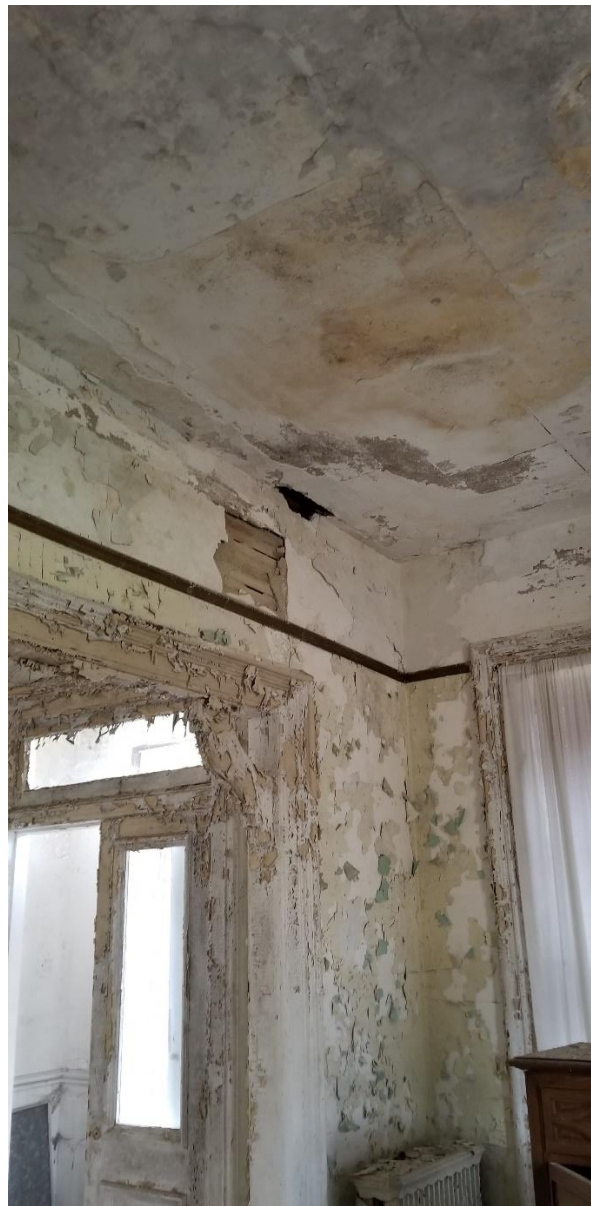
30. Staining on ceiling due to water Infiltration from roof leaks
