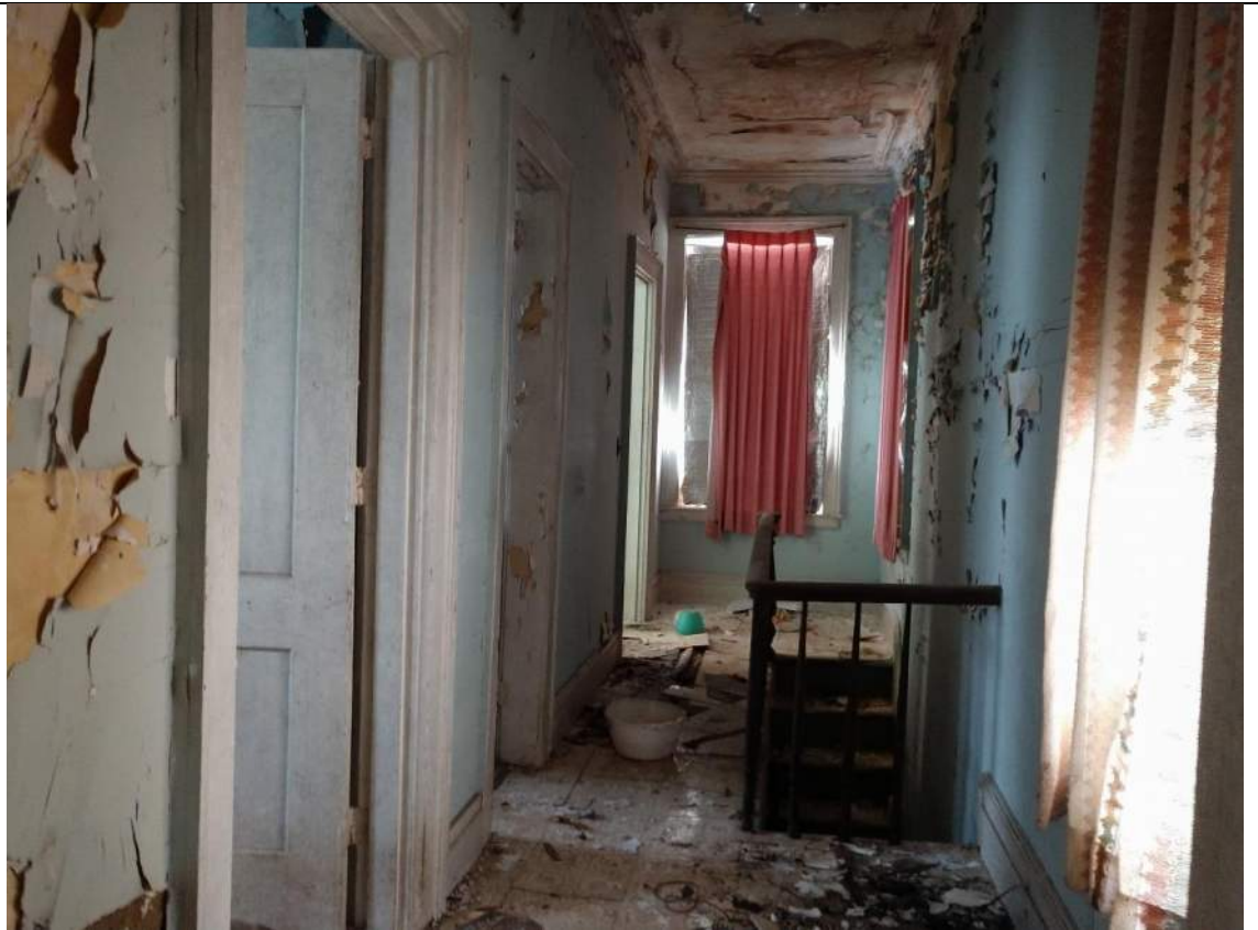
63. Hall to Rooms above kitchen, Rooms 208-206. Due to the collapsing floor, this area was too dangerous to assess.
