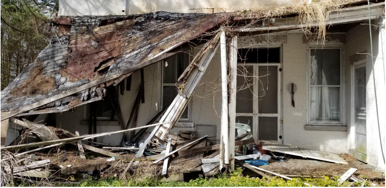
16. Collapsed porch roof on south elevation with debris
