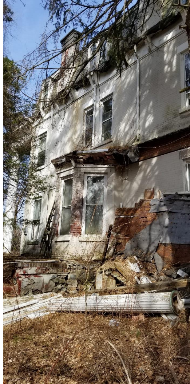
11. Collapsed porch roof on west elevation; damage to roof over window bay
