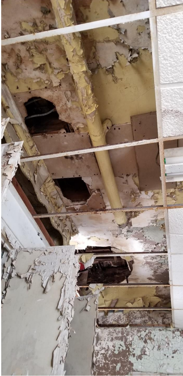
27. Ceiling damage due to leaking roof above over kitchen area
