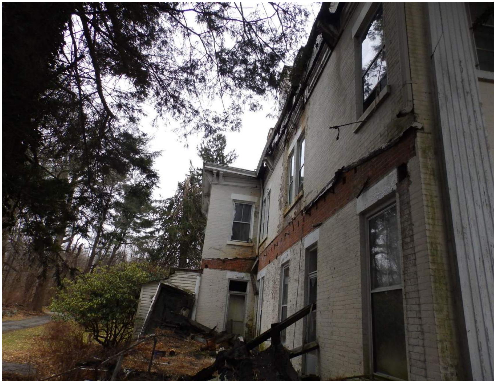
12. Detail of the eastern elevation. Note shed addition to the eastern side of kitchen addition.
