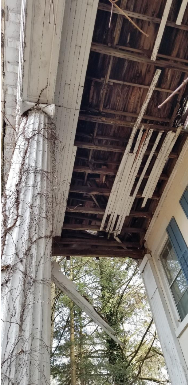
7. Deterioration of portico roof at front (north) elevation
