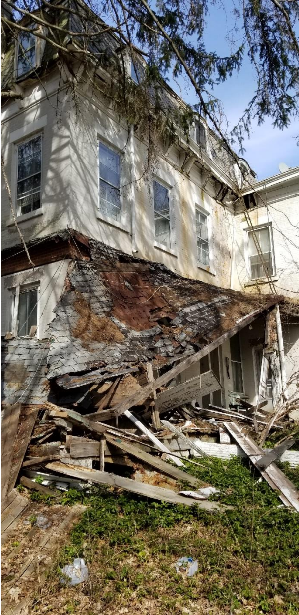
14. Collapsed porch roof on south elevation with debris
