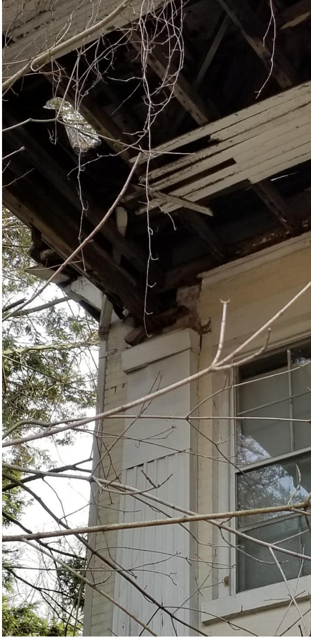
5. Deterioration of portico roof at front (north) elevation
