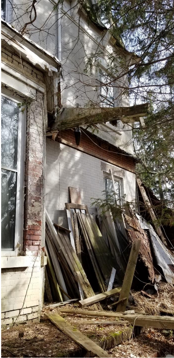
10. Collapsed porch roof on west elevation; debris
