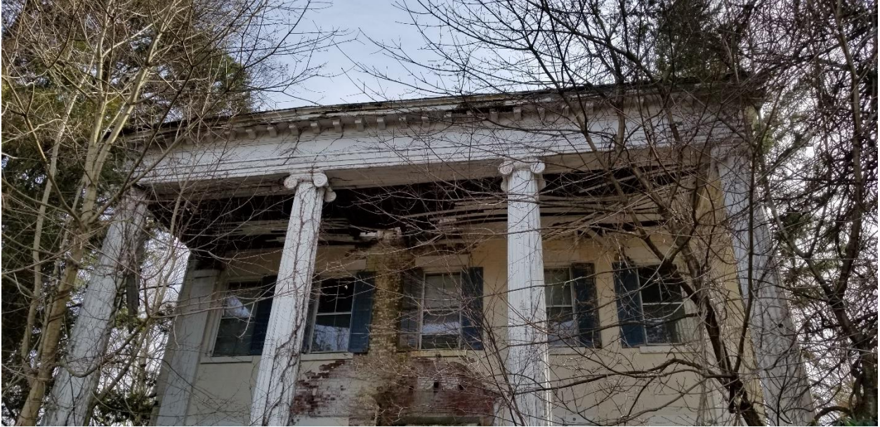
3. Deterioration of portico roof at front (north) elevation
