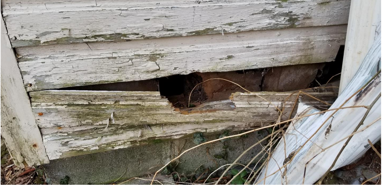
21. Deterioration of building addition area on southeast portion of structure
