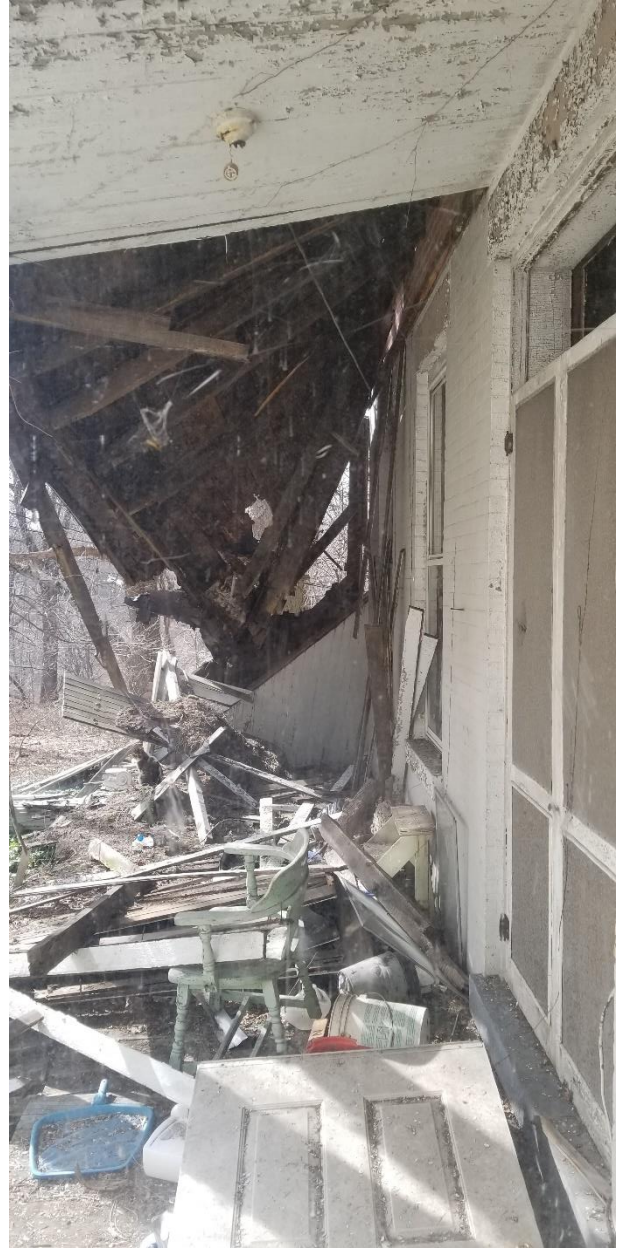
15. Collapsed porch roof on south elevation with debris
